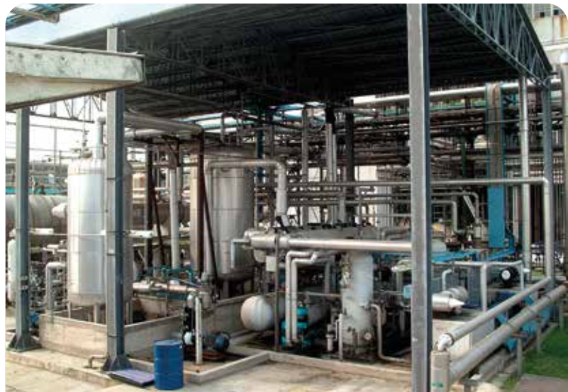
Refrigeration system for the production of antibiotics
